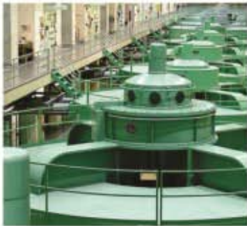
Captive Power Plant
